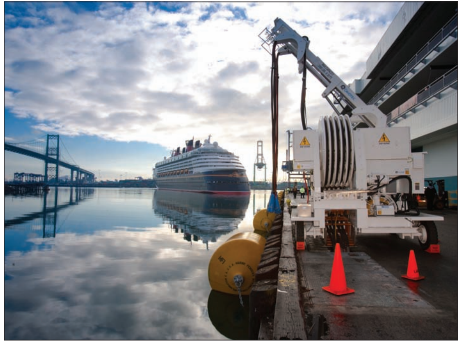
Disney cruise liner departs Port of Los Angeles following stop where AMP mobile unit (foreground) provided shoreside power.
